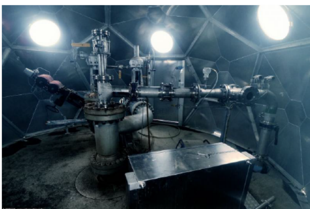
Interior, CarbFix2/Climeeworks CO 2 injection well, Hellisheiði, Iceland. © 2017 Adam Sébire . Used with permission.
