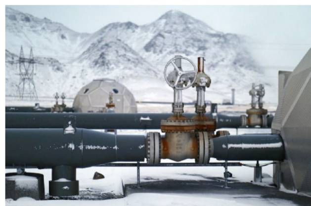
CarbFix2/Climeeworks injection wells, injecting CO 2 into the basalt below the Hengill volcano, Hellisheiði, Iceland. © 2017 Adam Sébire . Used with permission.
