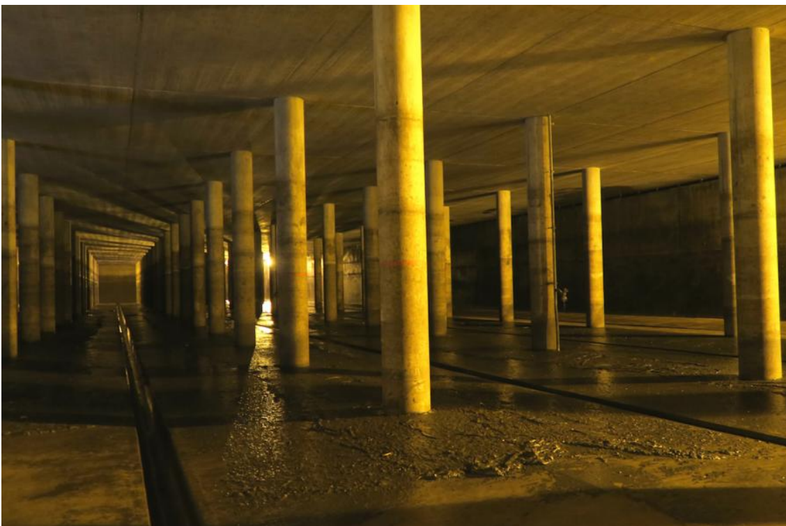
To ensure that wastewater does not flow into the Isar, enormous subterranean basins store excess water. Photos © Lisa Bauer. These works are licensed under a Creative Commons Attribution 4.0 International License.
