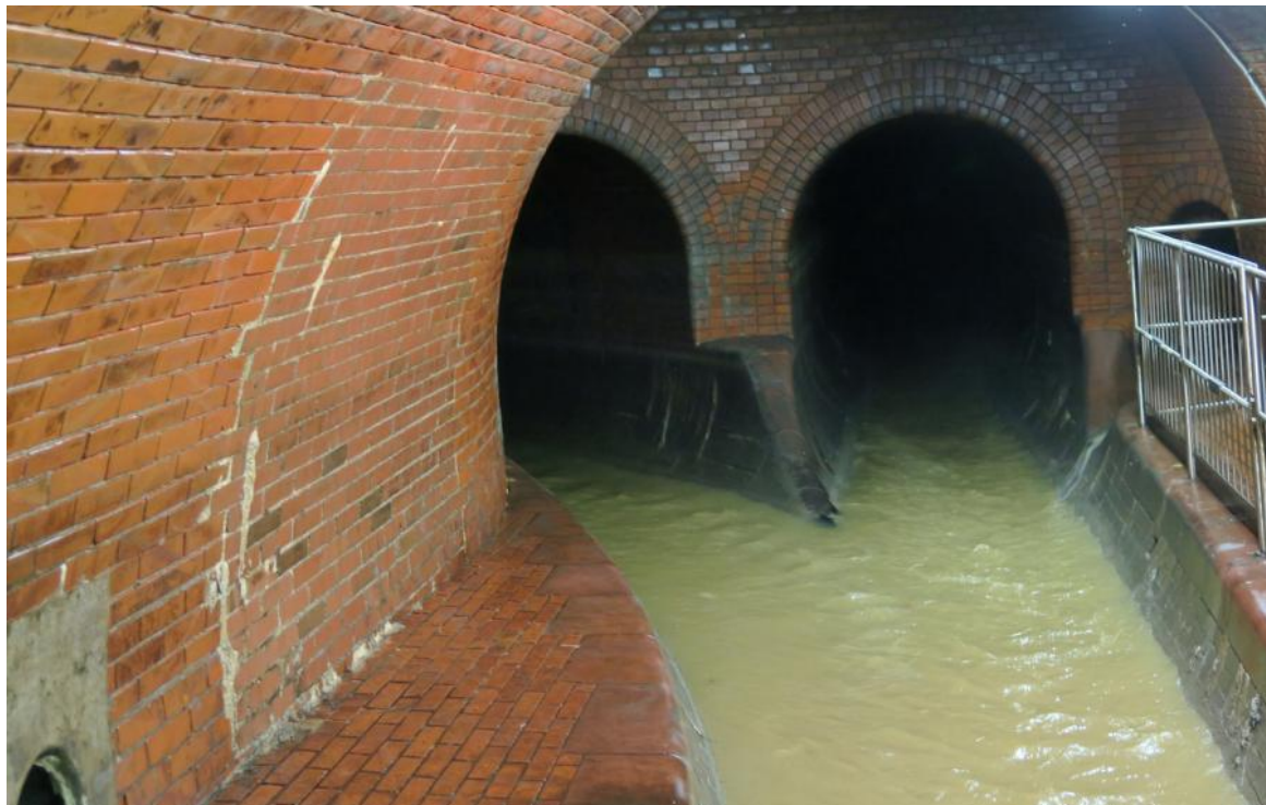
This masonry canal was built in 1912. Even today it drains wastewater from surrounding houses. Photos © Lisa Bauer. These works are licensed under a Creative Commons Attribution 4.0 International License.
