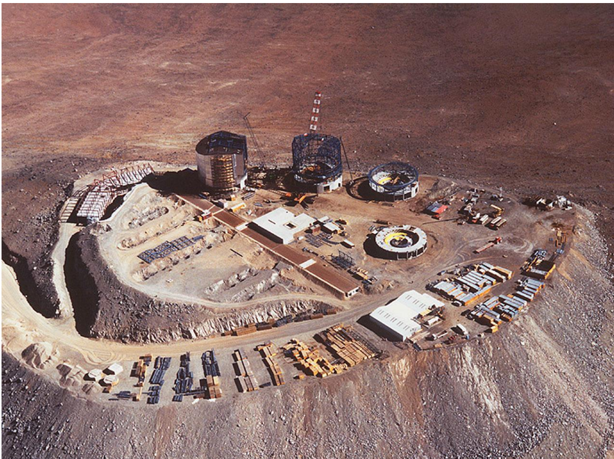
This image depicts the VLT construction site on Paranal from an altitude of about 3,000 meters. Unknown photographer, n.d.
