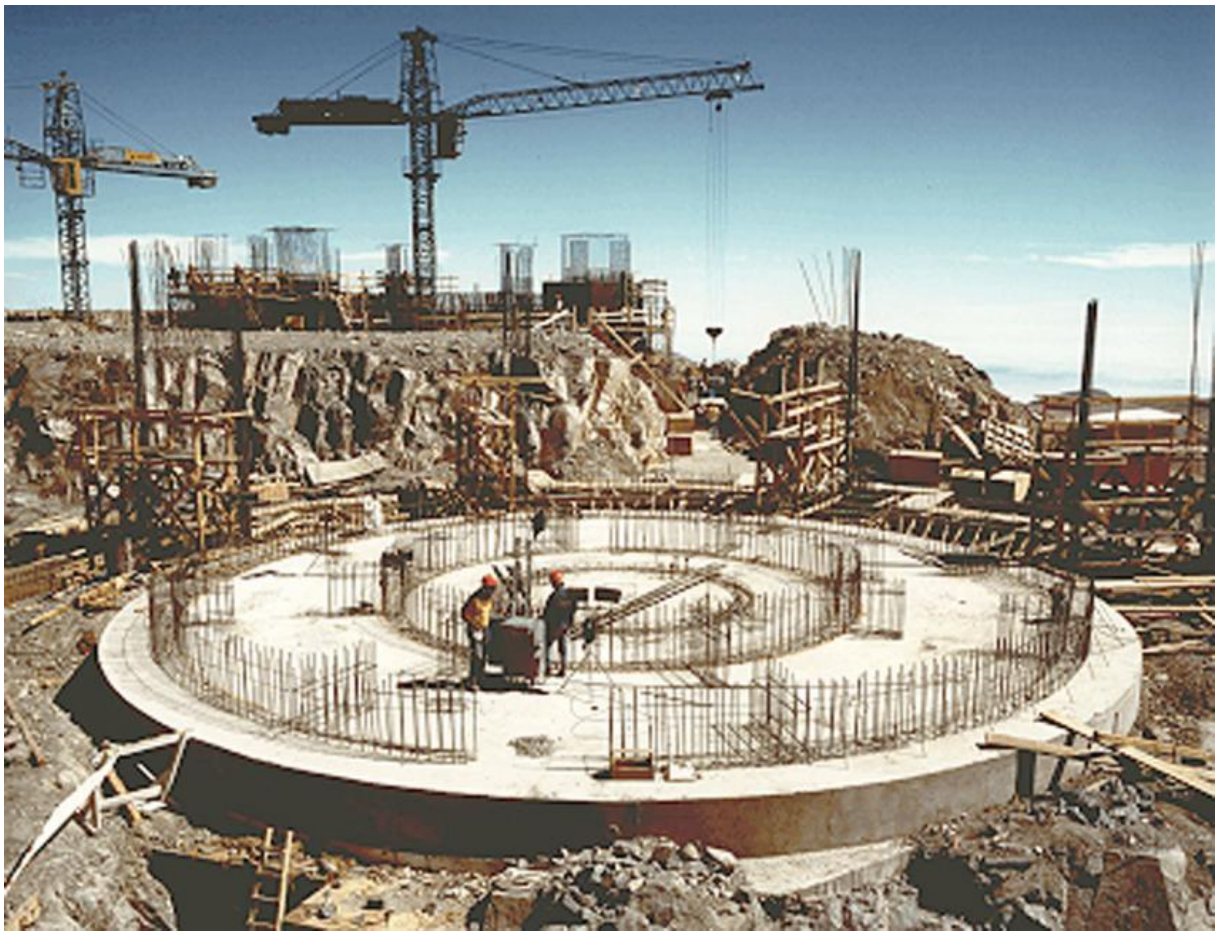
This photo was obtained in mid-September 1994 and shows the work at Cerro Paranal on the foundations for VLT Unit Telescopes no. 1 (background) and 2 (foreground). Unknown photographer, 1994.
